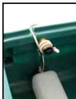
Frost protection heating cable wrapped around the valve
